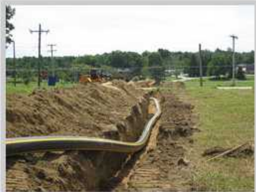
In areas without wetlands, open-cut methods were used to install the pipeline. Photo courtesy of R.H. White
